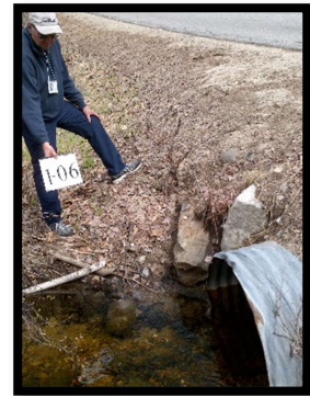
Documenting erosion during a watershed survey.
